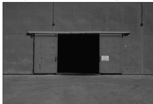
Figure 13-20. The large aircraft doors on facilities 1, 6, 16, 94, and 97 incorporate “pilot doors” for personnel and vehicular access.
