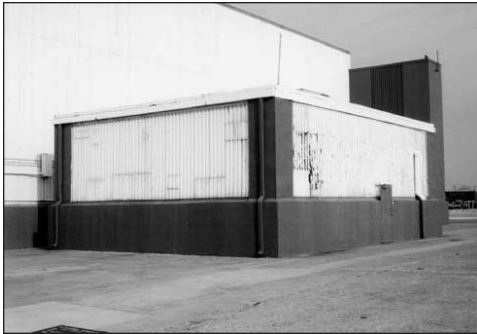
Figure 13-17. Concrete and box-ribbed steel siding are exterior materials used on historic facilities at NWIRP Dallas.
