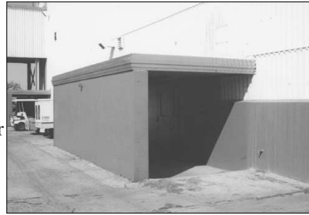
Figure 13-19. Concrete bomb baffles at entrances are an important character-defining feature of facilities 1, 6, and 7.
